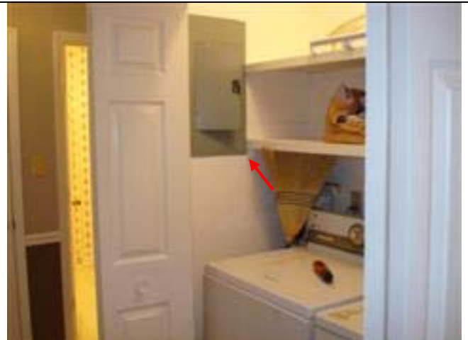
Electrical service panel has restricted access.
