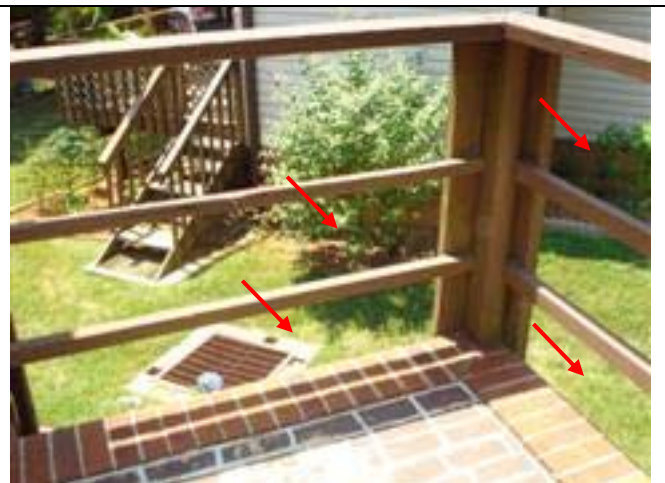
Right side porch railing openings are unsafe for children.
