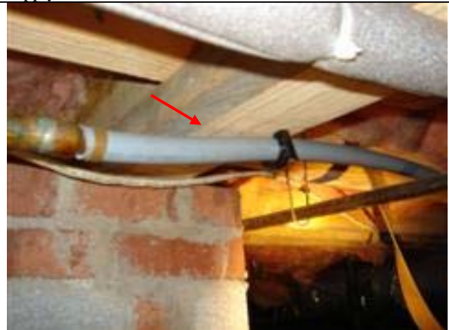
PB water supply tubing used in crawl space.
