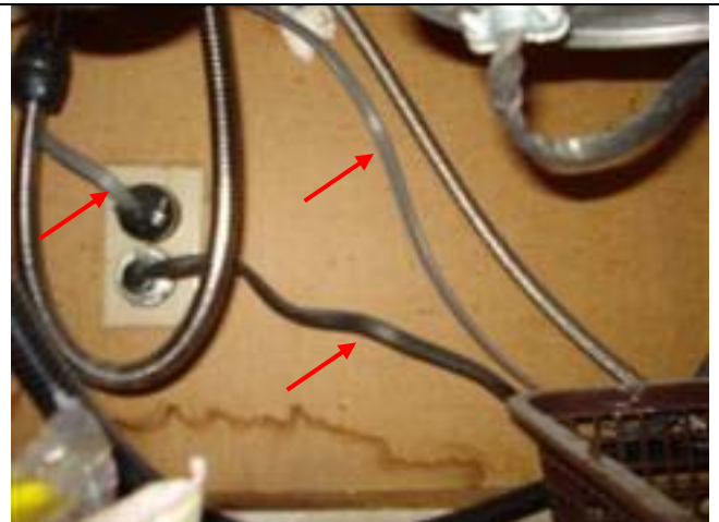
Wiring cables rated for use inside walls and conduit need protection from damage inside kitchen sink cabinet.
