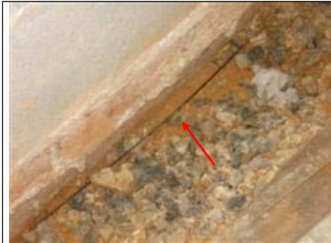
Evidence of previous water streaming along inside of foundation walls.
