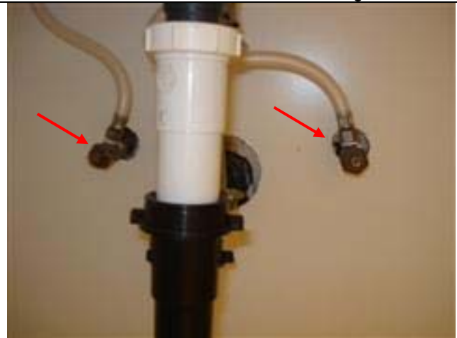
Gate valve handles missing for master bath lavatory water supply lines.
