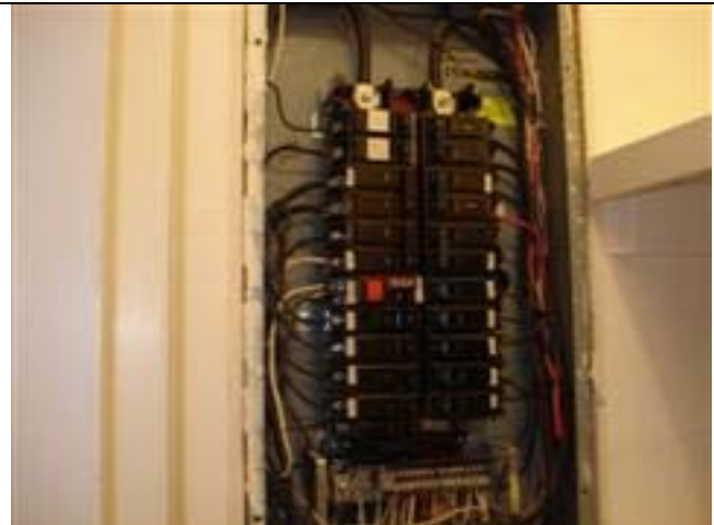
Dead front cover removed for inspection of electrical service panel.
