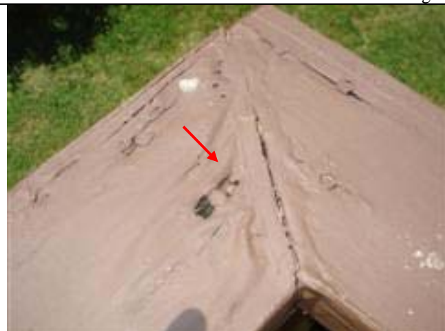
Wooden porch railing suffered moisture damage at right side.
