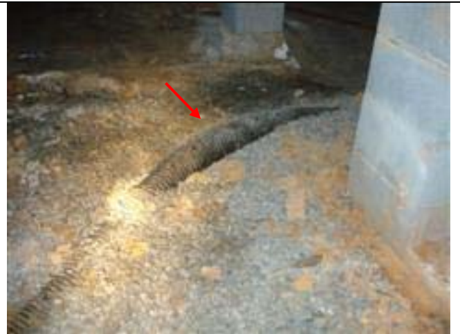
Crawl space drain conduits “porpoising” creates blockages in drain.
