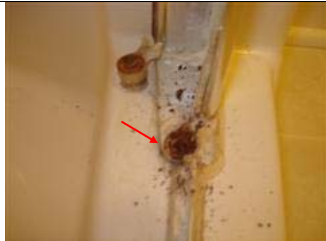
Shower door rusted at bottom hinge pin. Door fell off assembly when opened.
