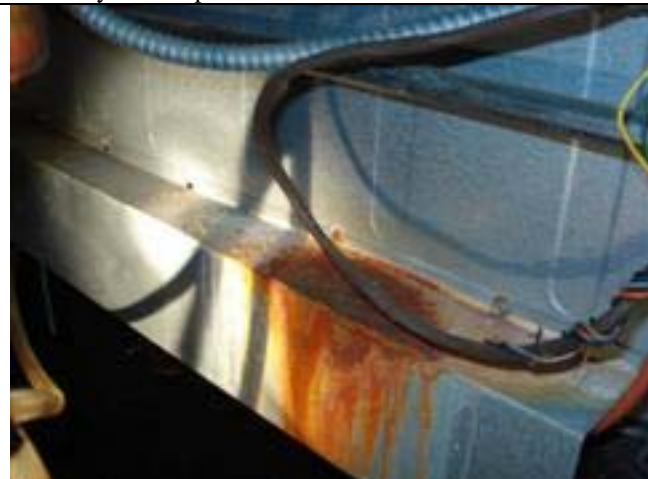
Leaking condensate drips onto flare shield of furnace.
