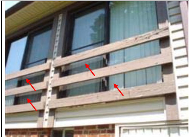
Railing openings at sliding doors are unsafe for children.
